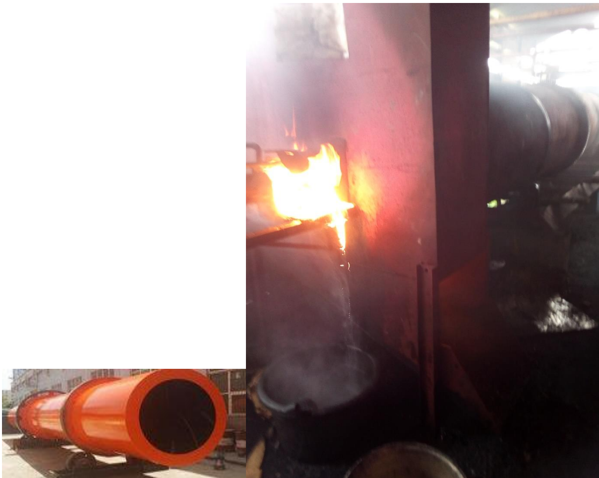
Figure 14 : Rotary kiln and burner running with used oil
